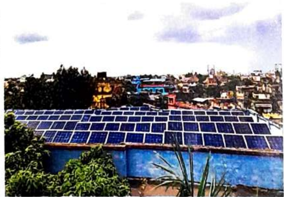
CAMPUS EQUIPPED WITH SOLAR PANELS
