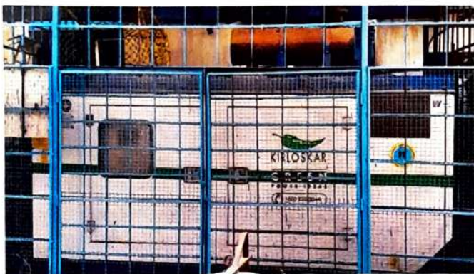
24X7 GENERATOR FACILITY
