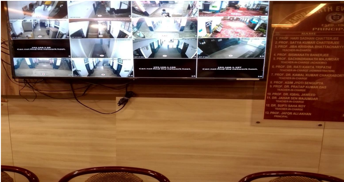
CCTV monitoring room
